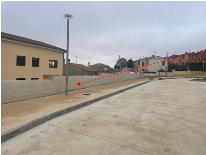
Remates de muro a comprobar
